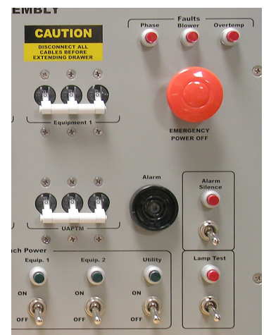
This partial view of an application-specific PDU control panel shows an EPO button, three-phase circuit breakers, and manual circuit switches.
